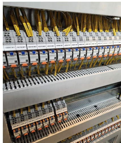
S7-PIR relay sockets installed in a Windhoff control cabinet
