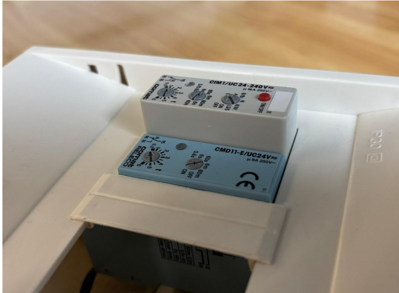
CMD (blue) and CIM1 (grey) in the sub-distribution board
